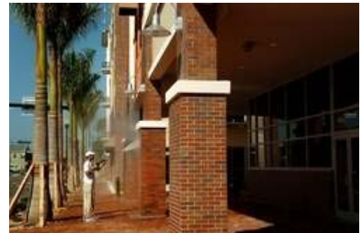
STAFF PHOTO / E. SKYLAR LITHERLAND A worker pressure washes the exterior of the new four-story city-owned Herald Court Centre parking garage in downtown Punta Gorda .
